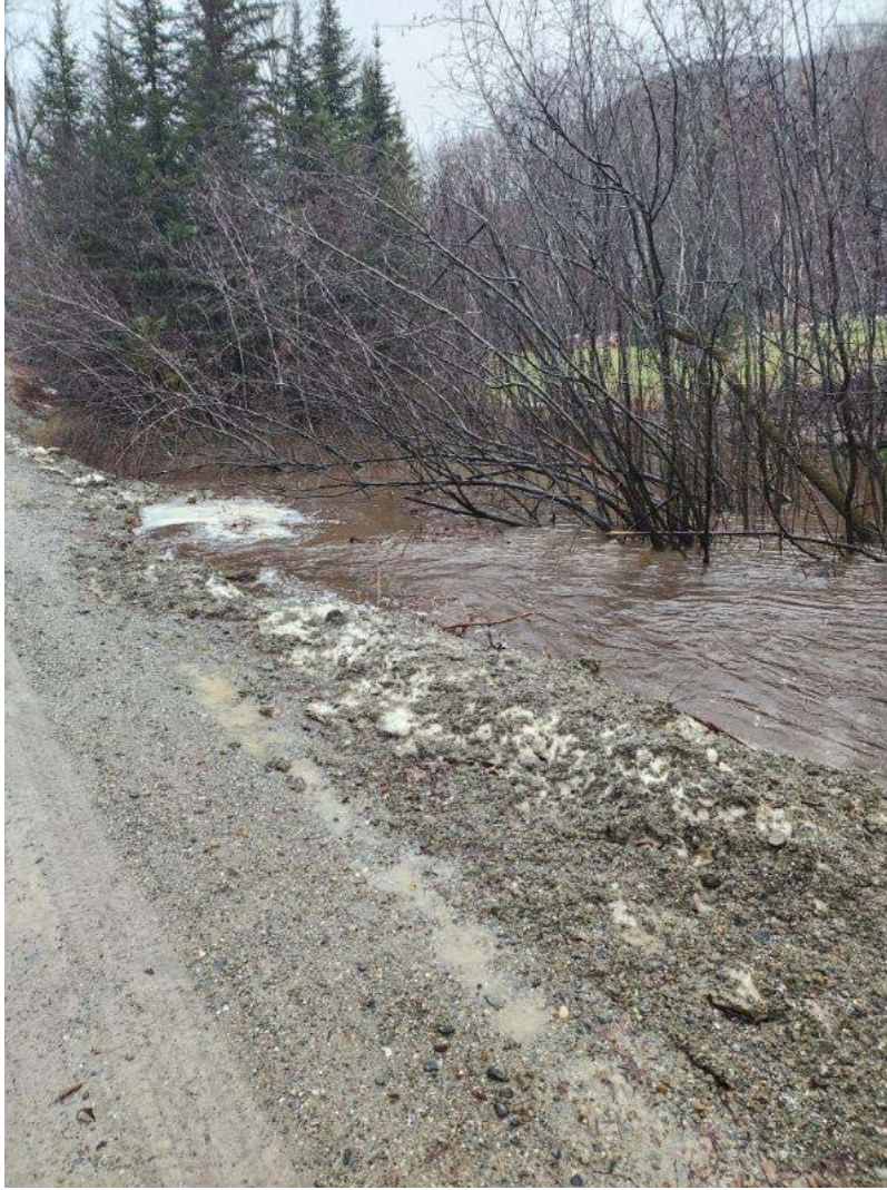
Segment 142058 Looking Northeast – white foamy area is the inlet of the culvert. This is during the heavy rain on Monday 12/18
